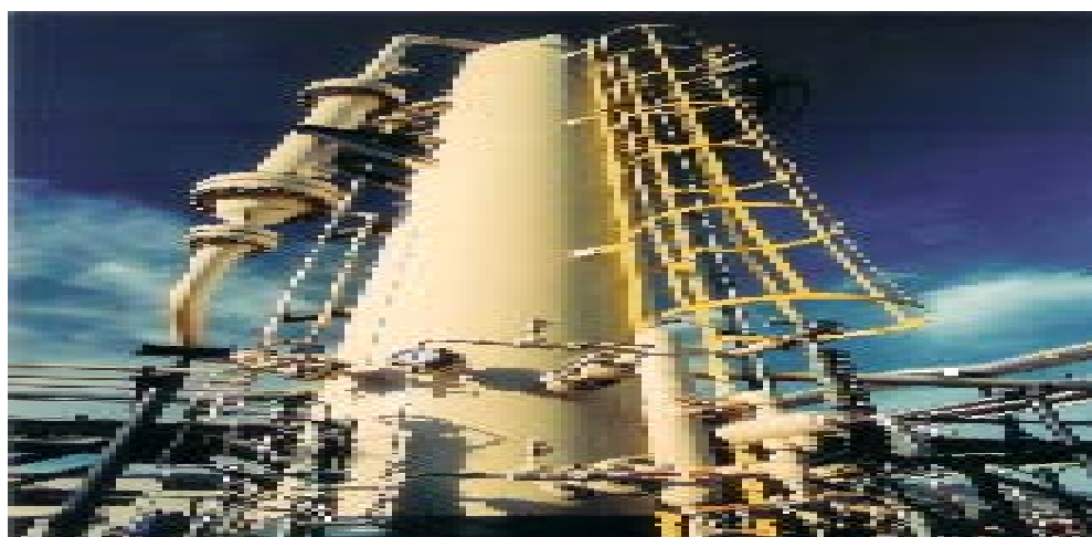
Hydrocarbon Processing Facilities Tal Block
